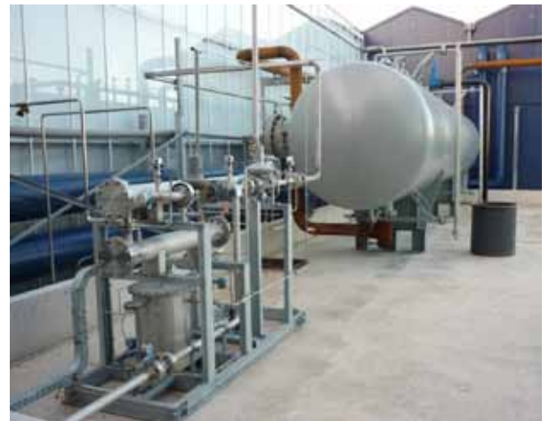
Geothermal drying & reducing installation
